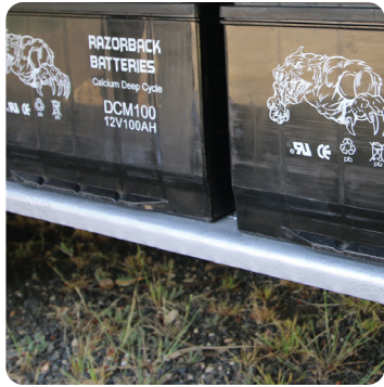
2 x 120amp AGM Batteries
